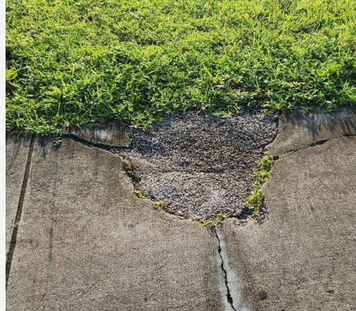
Cracking in sidewalk
