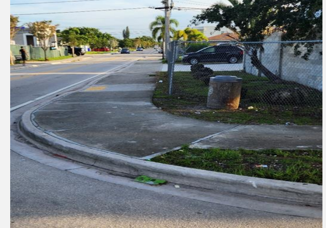
Missing curb ramp
