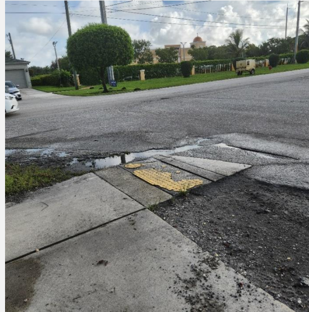
Damaged ADA Curb Ramp
