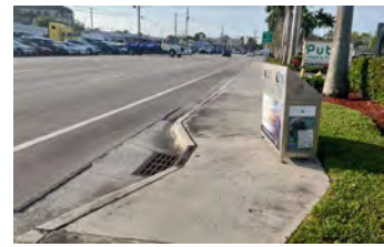
West ROW: Sidewalk is recessed at location of storm drains
