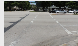
Faded Pavement Markings
