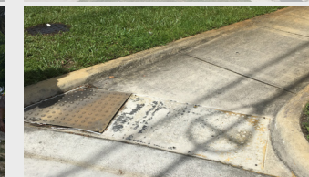
Poor ADA Compliance
