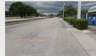
Excessive Pavement Width
