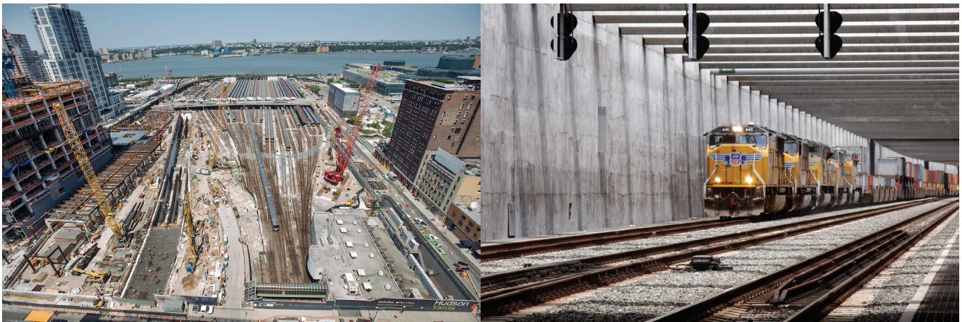
Advance preparations for proposed new trans-Hudson River tunnels (far left in photo) are part of the Hudson Yards project in New York City. The existing tunnels are an incredibly critical link in the nation’s rail system and for the New York regional economy. Photo by the Metropolitan Transportation Authority. https://www.flickr.com/photos/mtaphotos/14794824672
